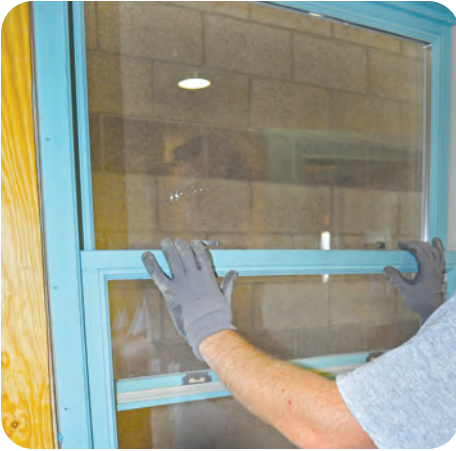
7. Ensure window is operational
